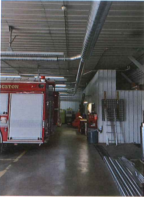
Overhead Piping That Mechanically Vents Exhaust Outside The Building
